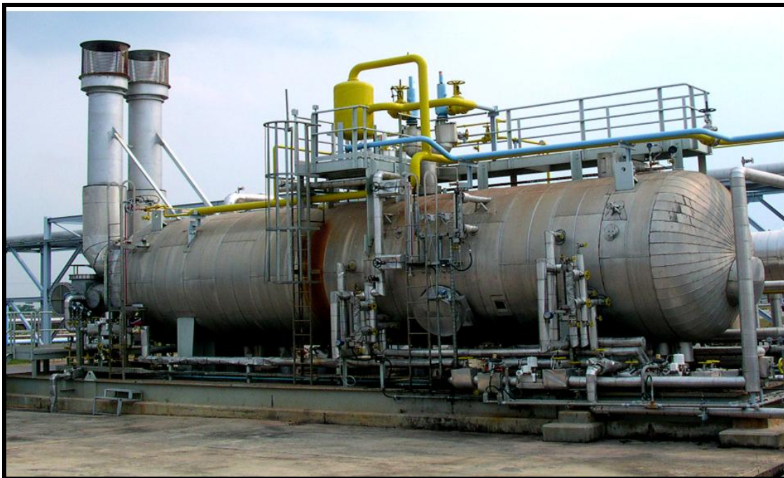
Gambar : Heater Treater
